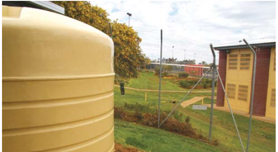
> Large rainwater tanks installed at Junee Correctional Centre form part of the centre's environmental management plan.
